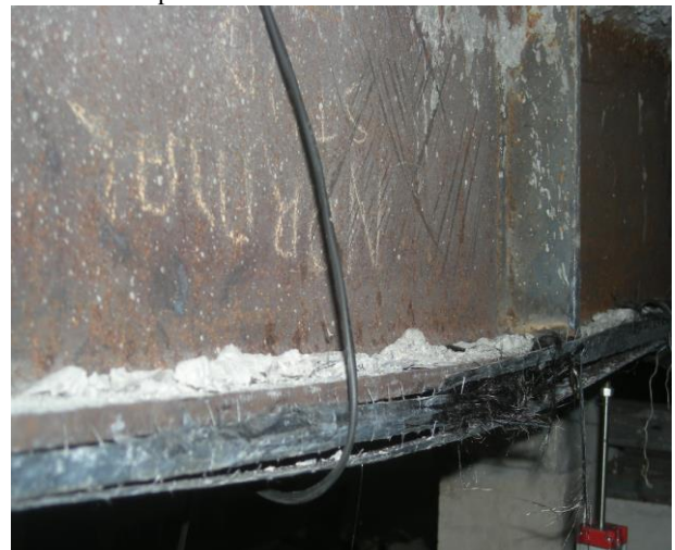
Figure 15. Rupture at edges and de-bonding of CFRP from steel in CBW2CFRP sample
