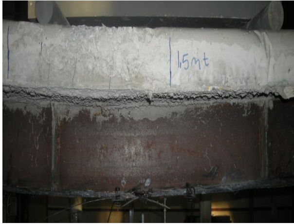
Figure 16. Shear cracks near the loading point
